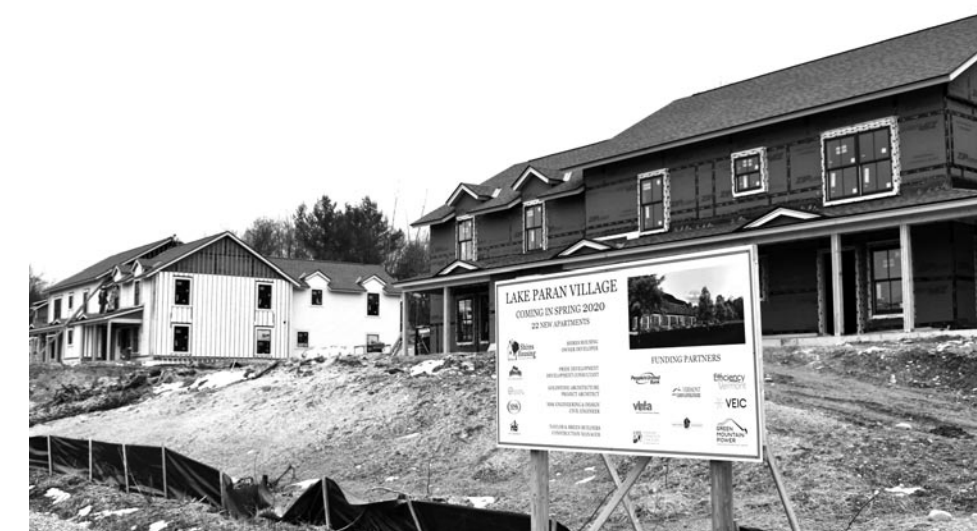
(above) Construction at Lake Paran Village – (top) work at East Branch Farms
